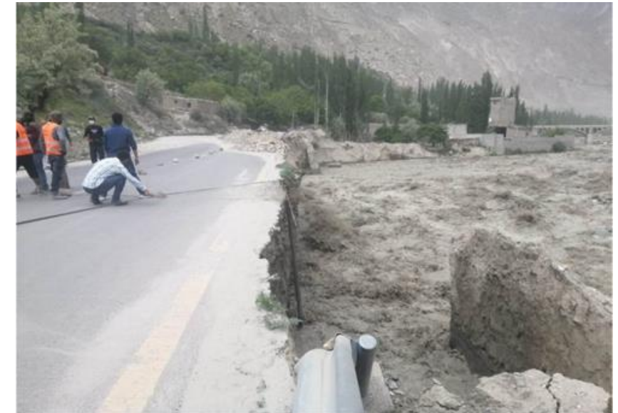
Damage of major GLOF event on Shishper glacier on the infrastructure in Pakistan in May.
